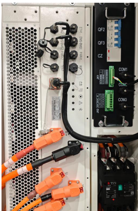
Figure 7-5 Power cable and terminal
